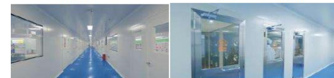
Air Shower Room
